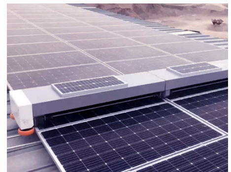
Solar panel cleaning Robot
